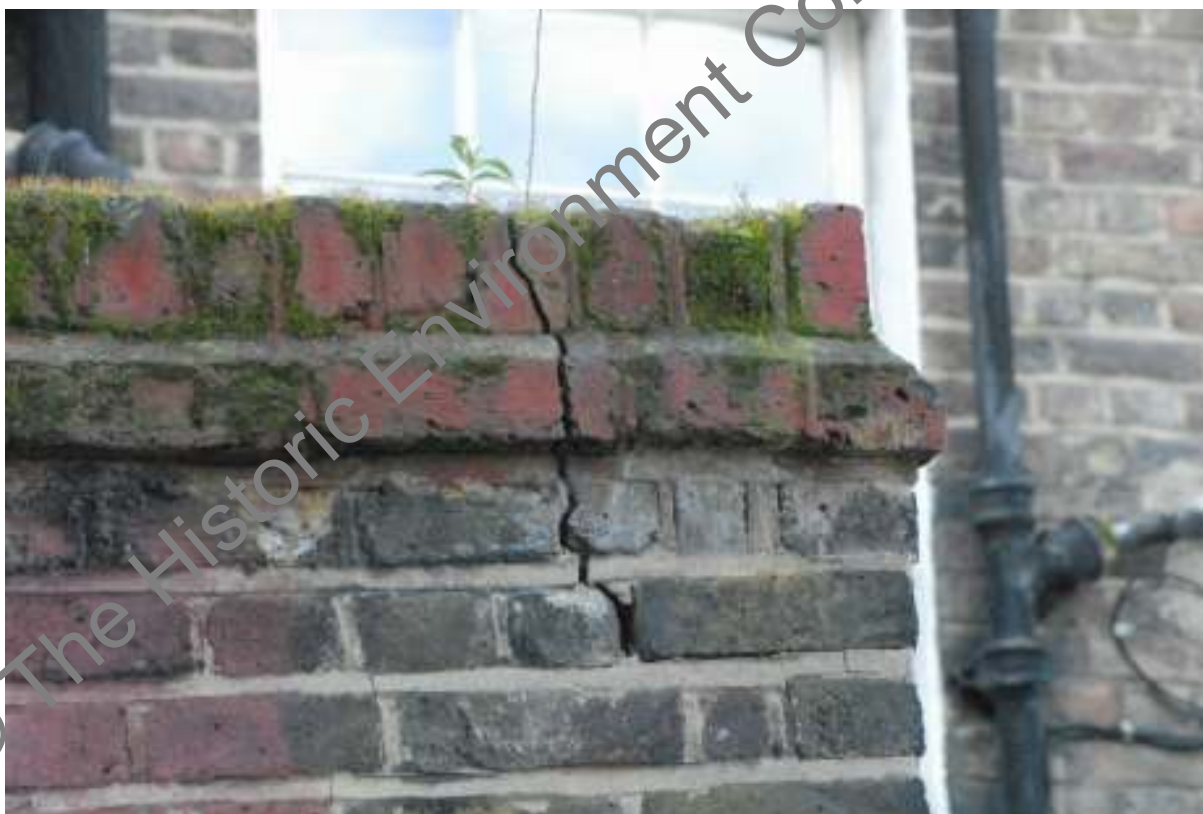
Plate27 Structural Instability rear extension
