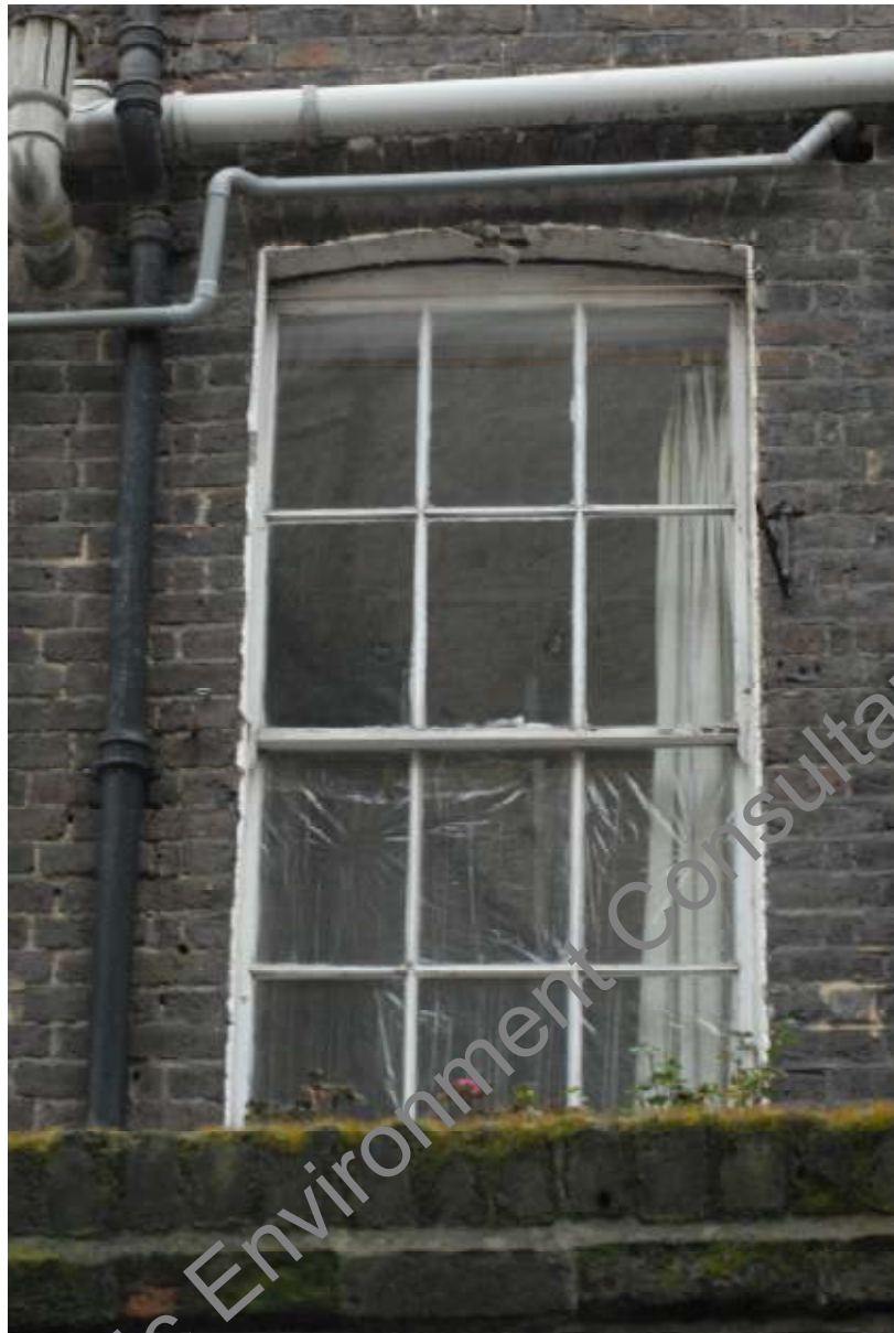
Plate34 The First Floor Kitchen Window clearly a none Georgian Form.
