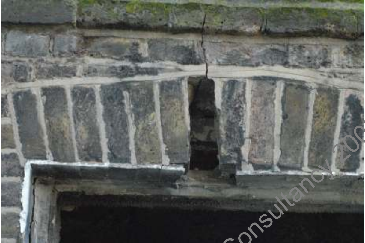
Plate28 Structural Instability Rear Extension
