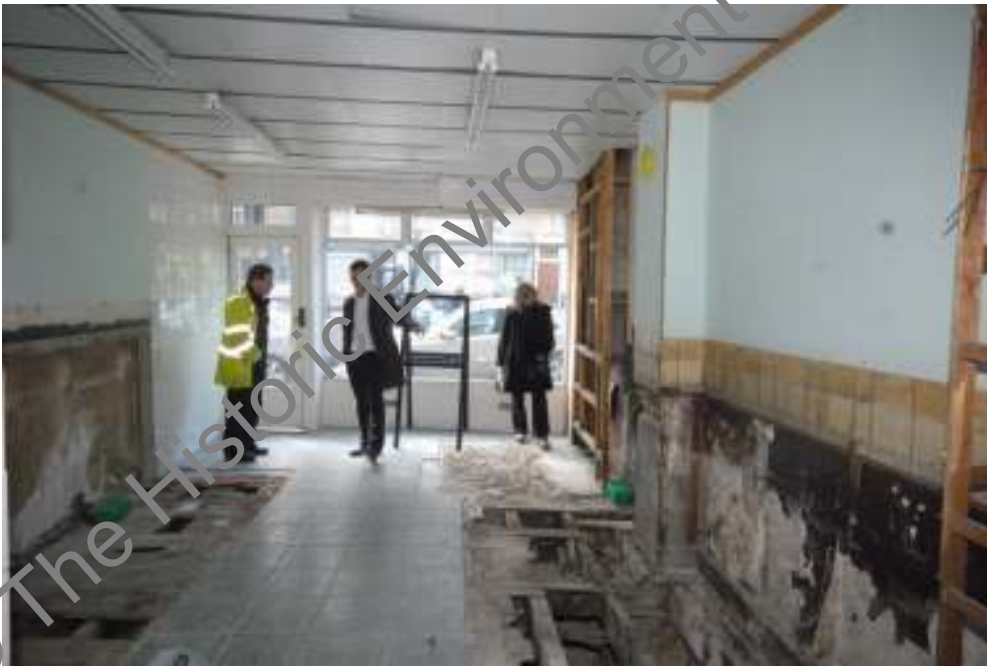
Plate29 Missing Floor boards etc ground floor
