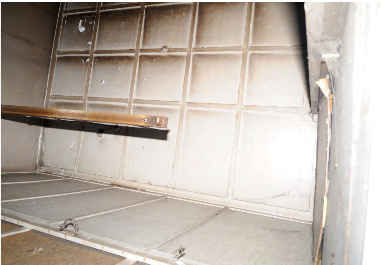
Plate 47: Detail of ceiling, northwest room, showing smoke damage The ceiling in this part of the room appears to be a 20 th century suspended ceiling.
