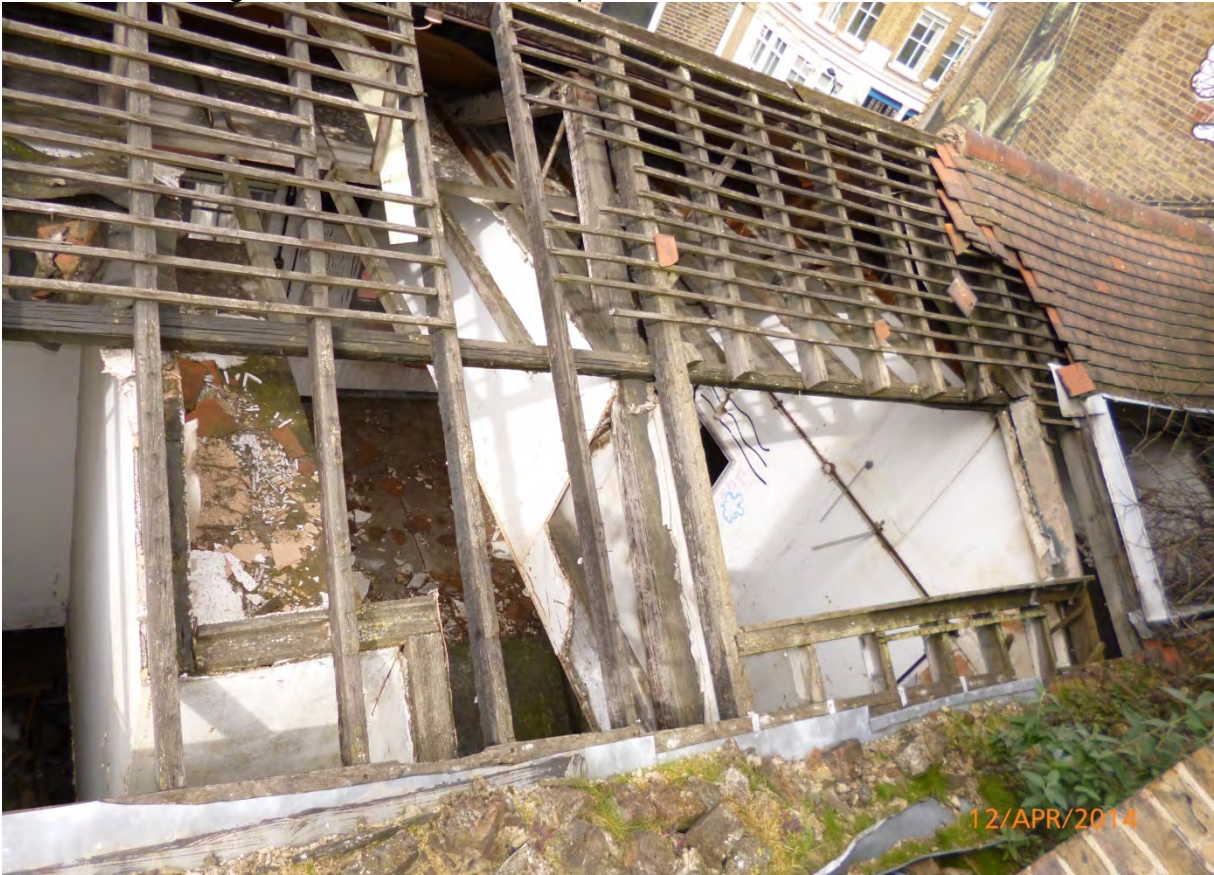
Plate 65: Absent roof covering, building to rear
