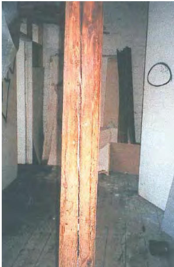
Plate 58: Split in timber post, 3rd Floor (Shaya 2000)
