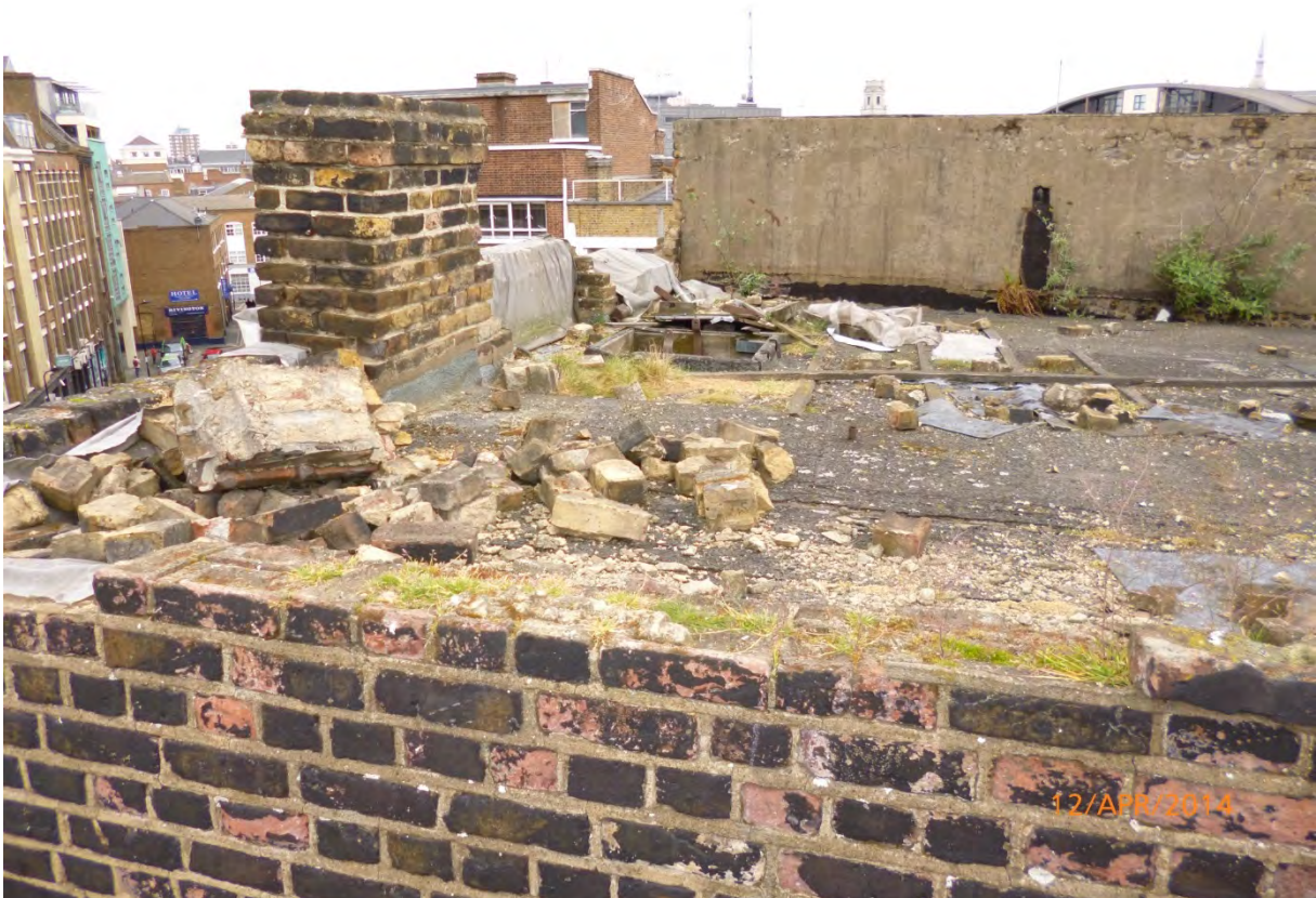
Plate 20: Structural damage to the roof of 63 Great Eastern Street
