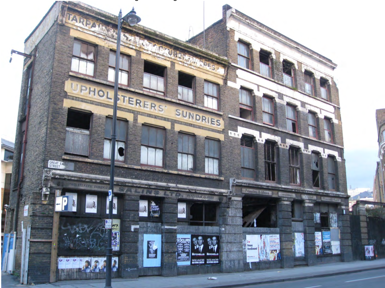
Plate 7: The northeast façade in 2009 prior to the installation of scaffolding 61 is a building of three floors with a parapet with corbels at either end.
