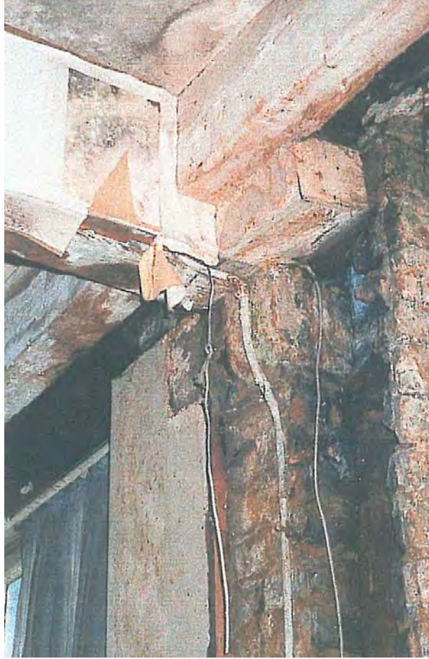
Plate 57: Detail of main and secondary beams at corbel junction, 3rd floor (Shaya 2000)
