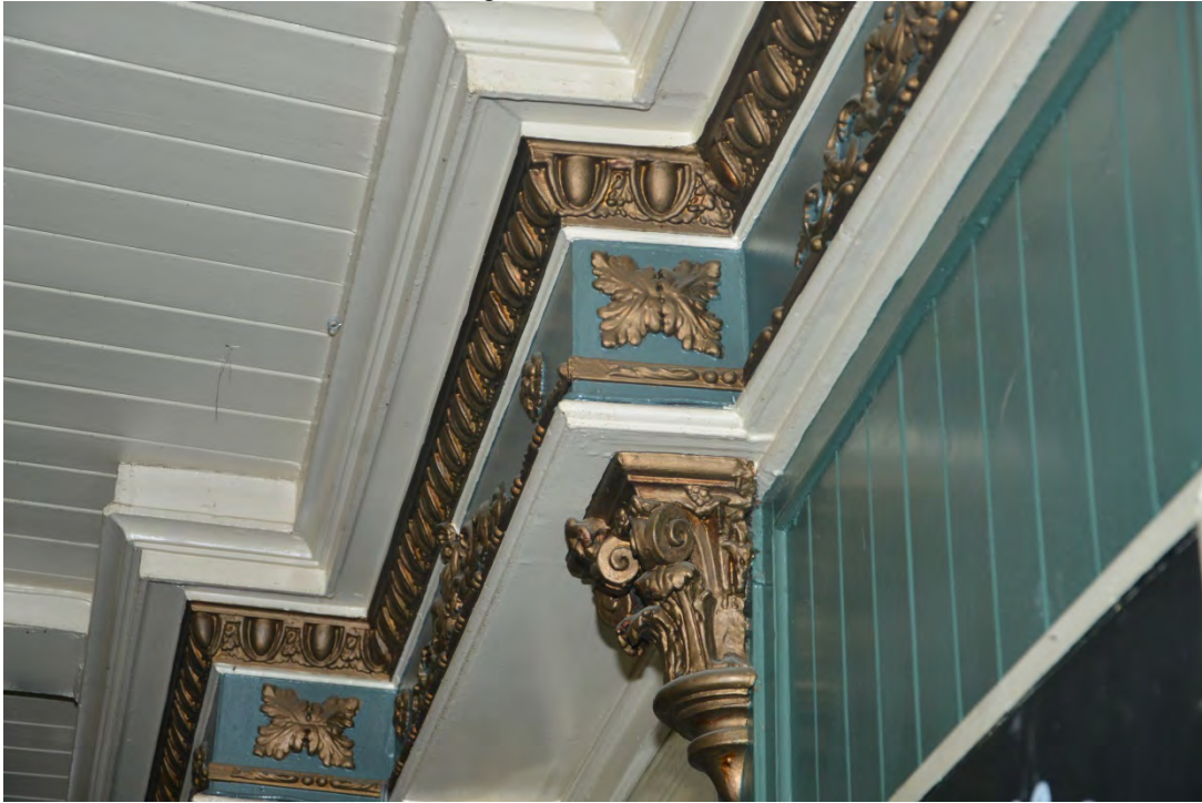
Plate 48: Mouldings to be refurbished and repainted
