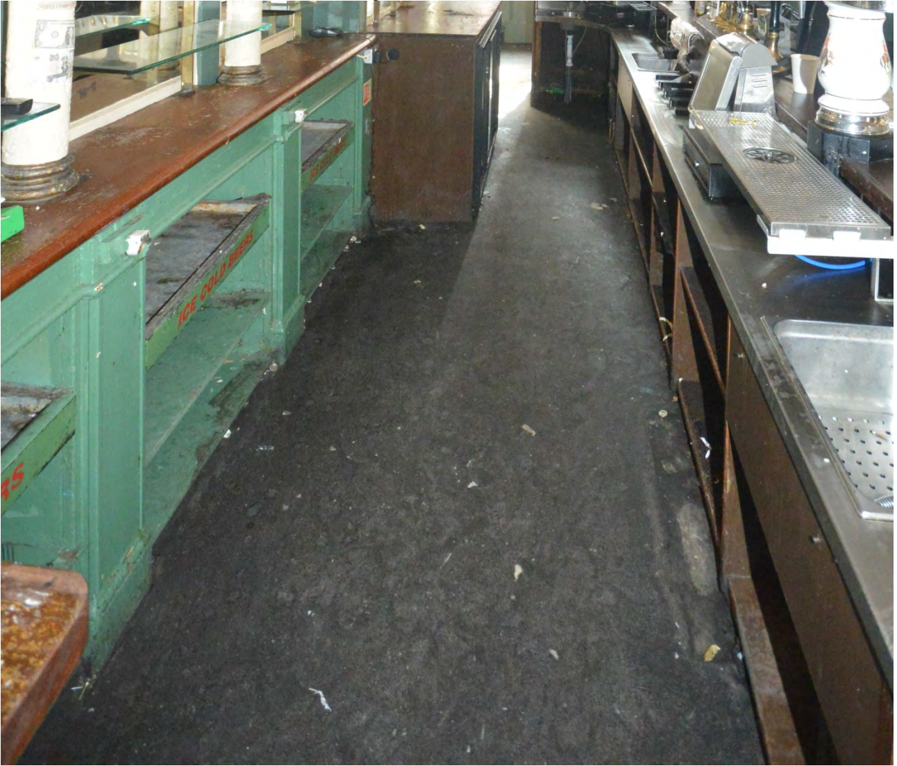
Plate 40: Flooring to be replaced
