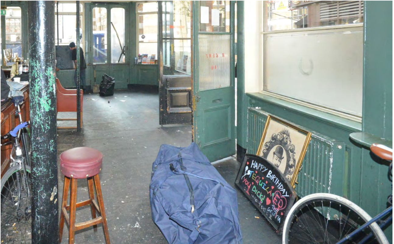
Plate 38: Flooring to be replaced
