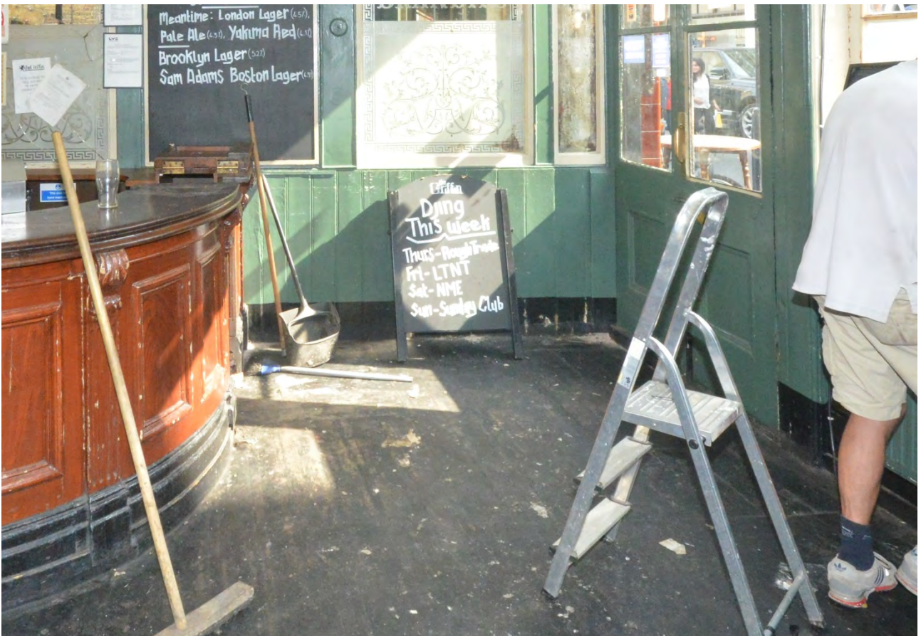
Plate 39: Flooring to be replaced
