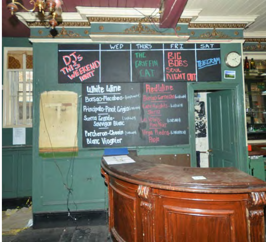
Plate 32: The left hand half of this partition wall is to be removed
