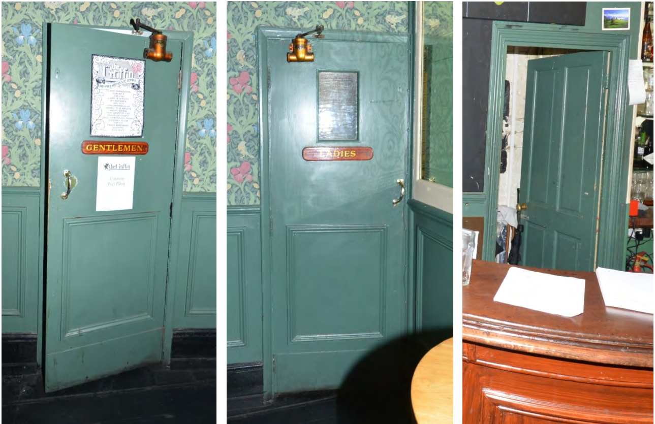
Plate 45: Doors to be replaced
