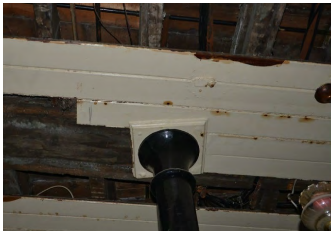
Plate 5: Lath & plaster marks revealed beneath tongue and groove
