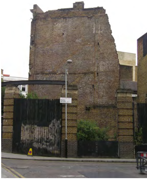
DP 5 Remains of 65 Great Eastern Street and gable end of 63 Great Eastern Street looking south-east
