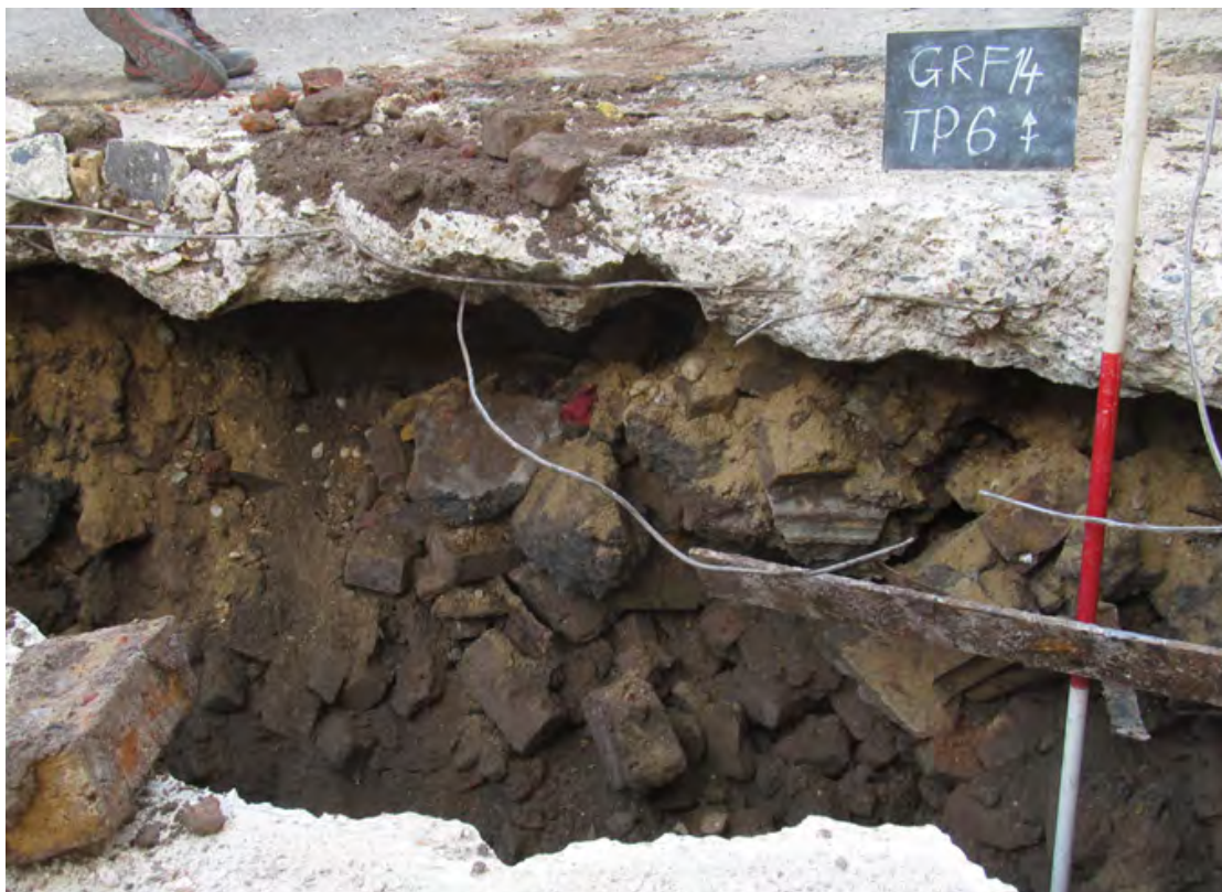
Plate 14: TP.6 – north section, showing brick wall underneath the concrete surface, looking north
