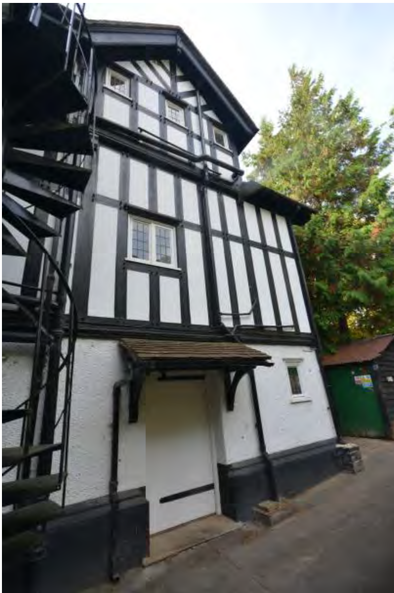
Plate 5: Northernmost gable, east elevation The above photograph is taken from lower ground floor level. A spiral fire escape staircase is visible to the left of the image, serving the ground and first floors of the northern part of the building.
