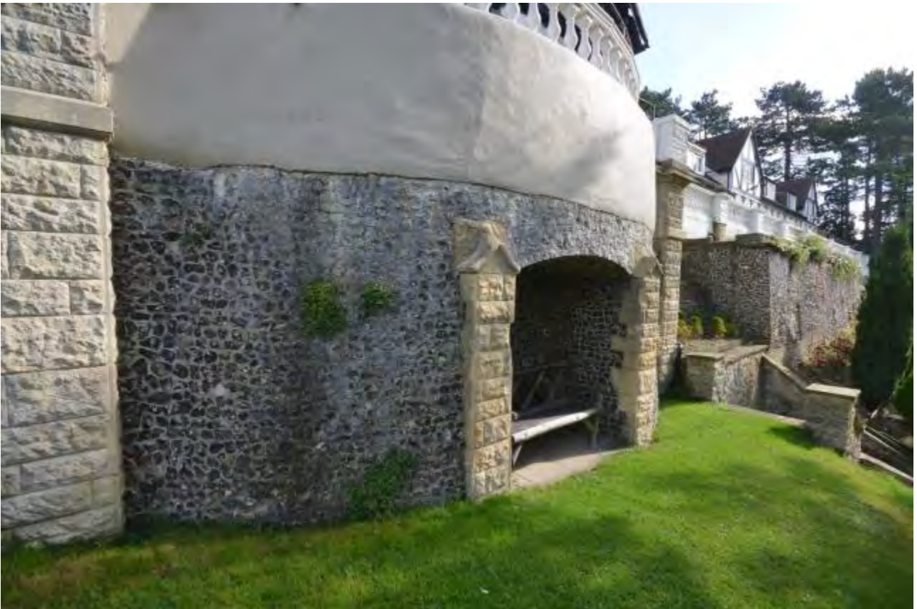
Plate 13: Detail of recessed seat in flint wall with stone piers, west elevation, Lakeside wing
