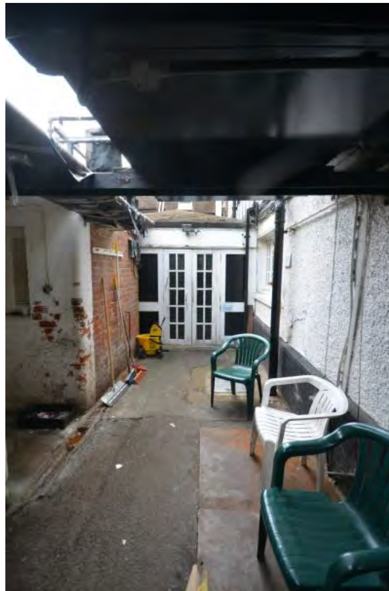
Plate 6: View south to kitchen doors, northern part of east side The above image is taken at lower ground floor level and shows the double doors into the kitchen area.
