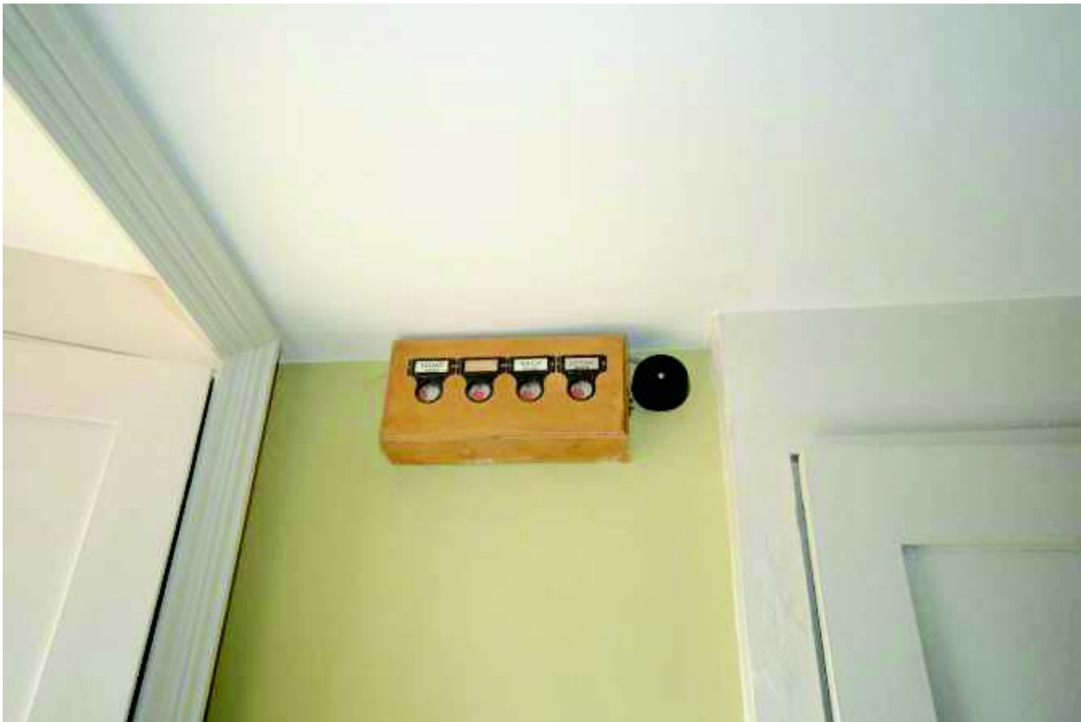
Plate 50: Detail of service bell and indicator board
