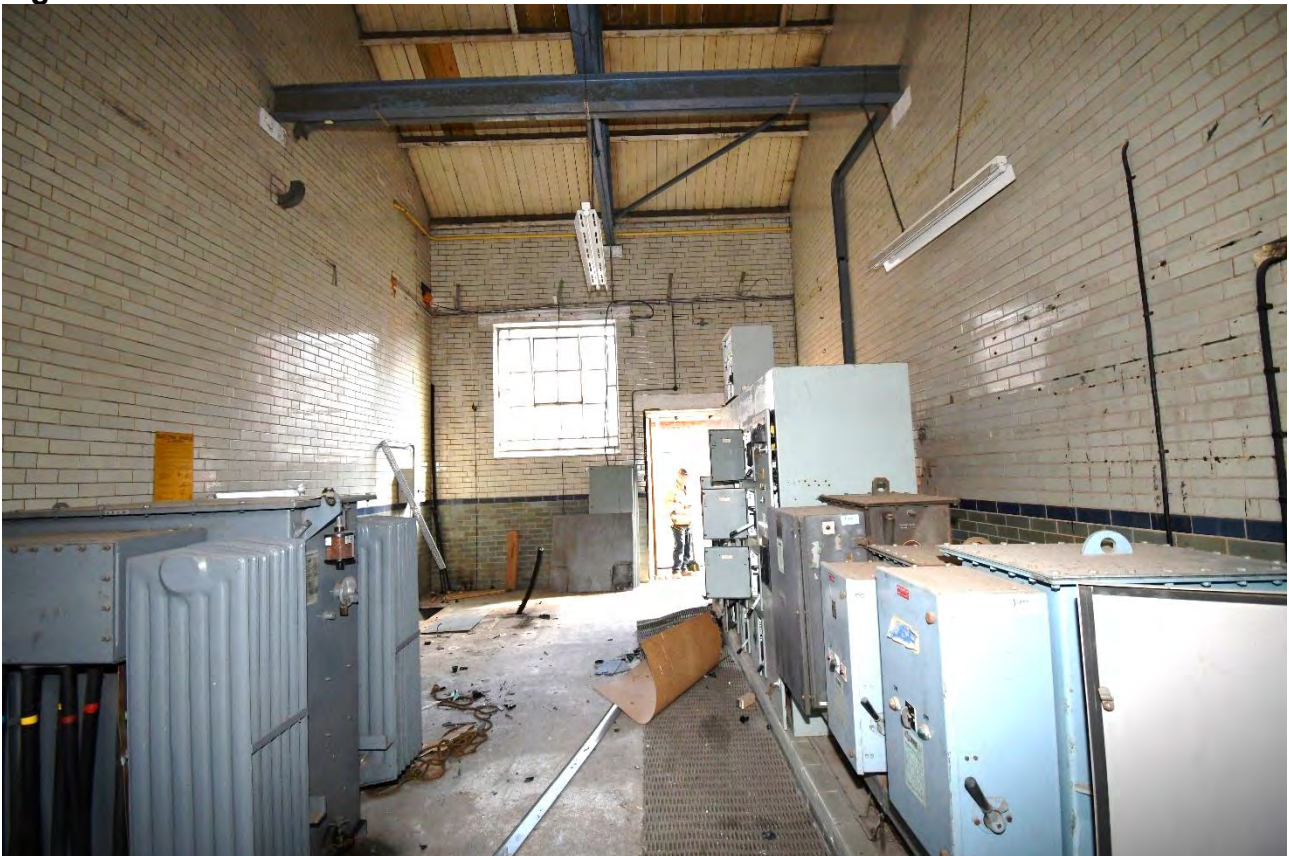
Plate 74: Power House Interior
