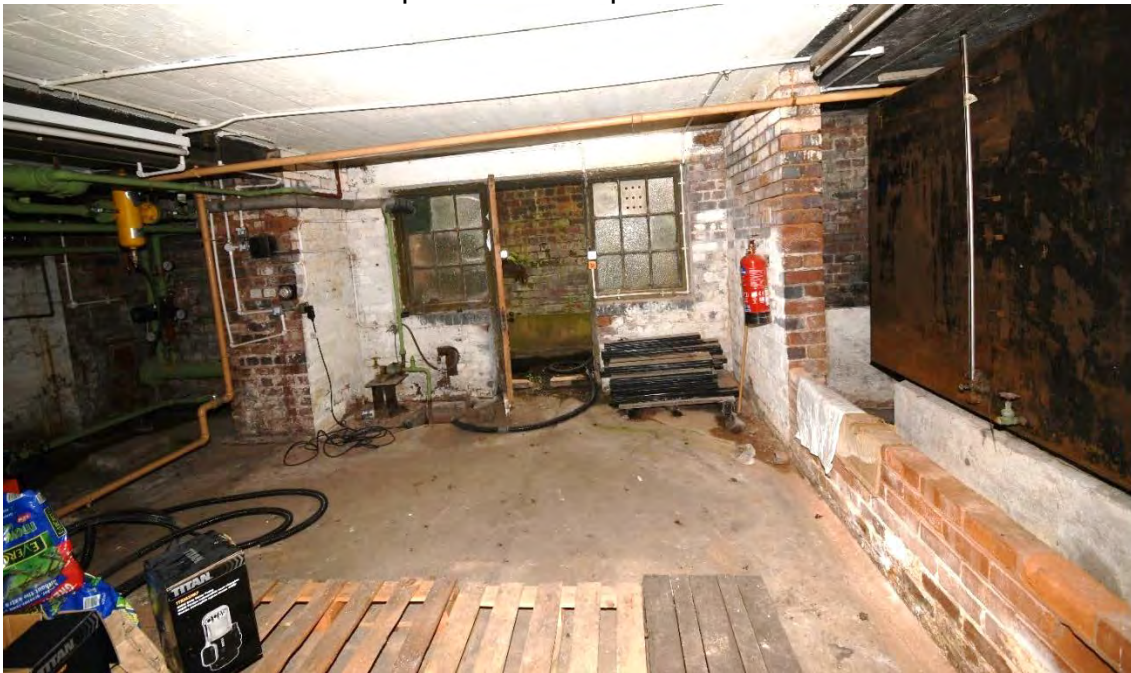
Plate 155: Plant Room Looking Northeast
