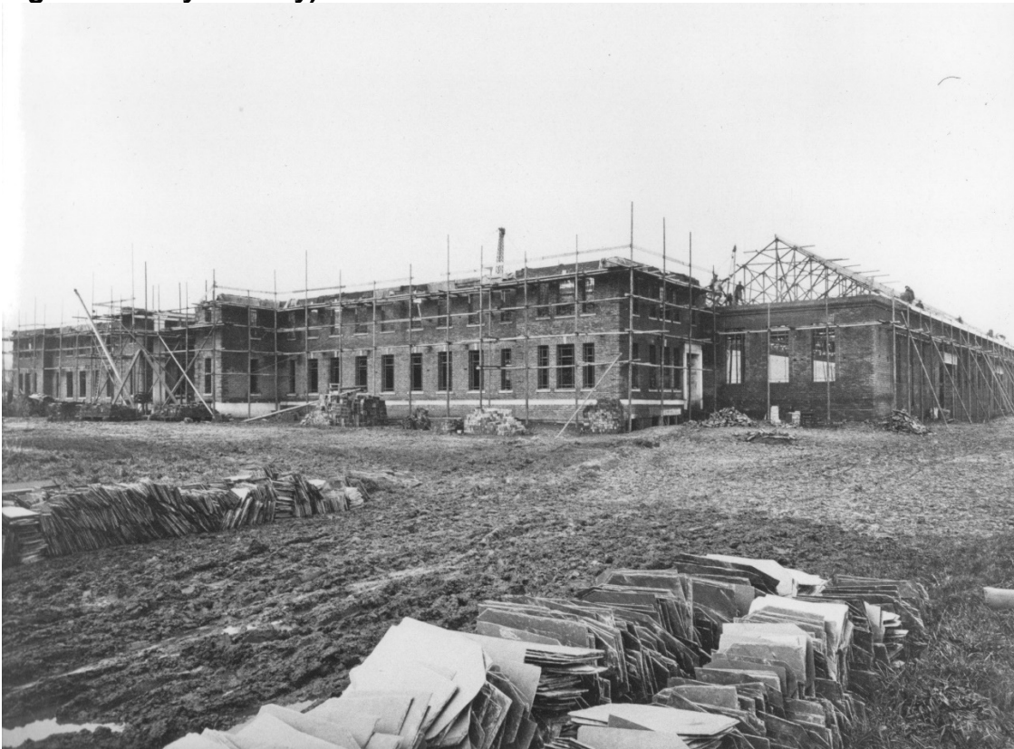
Plate 3: The northeast part of the building under construction, 1927 (Blue Bird Album, Romsley & Hunnington History Society)
