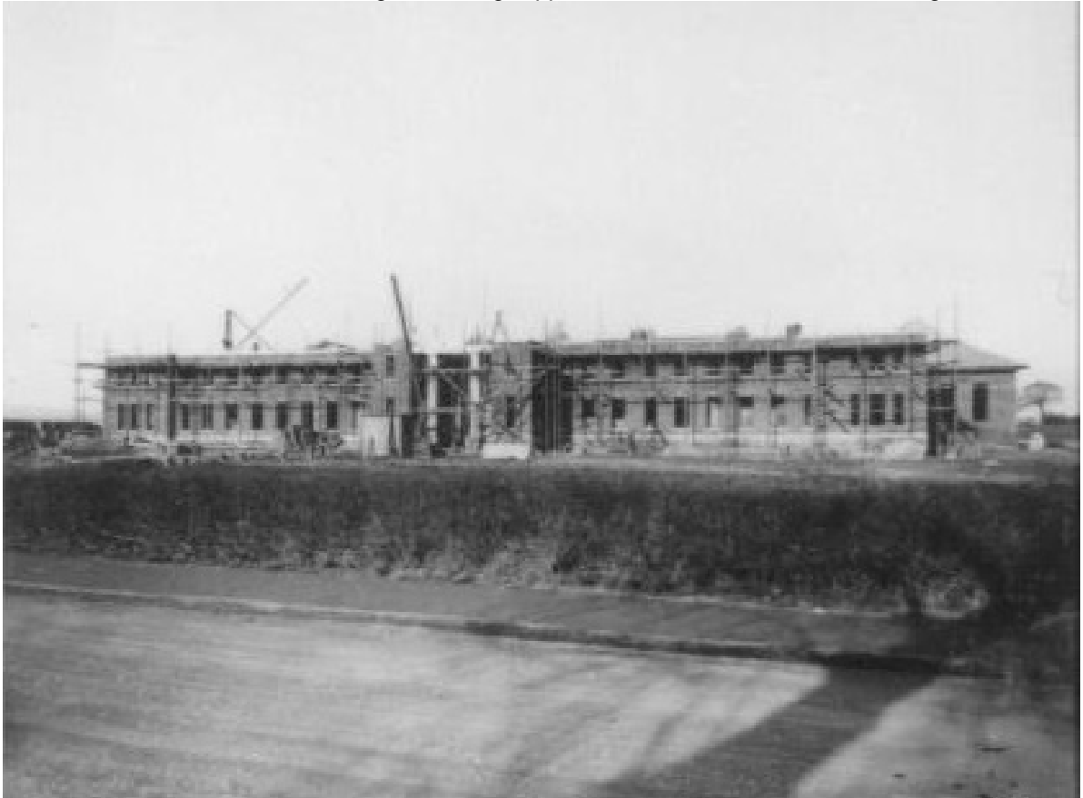
Plate 4: The southeast face of the building under construction, 1927 (Romsley & Hunnington History Society)
