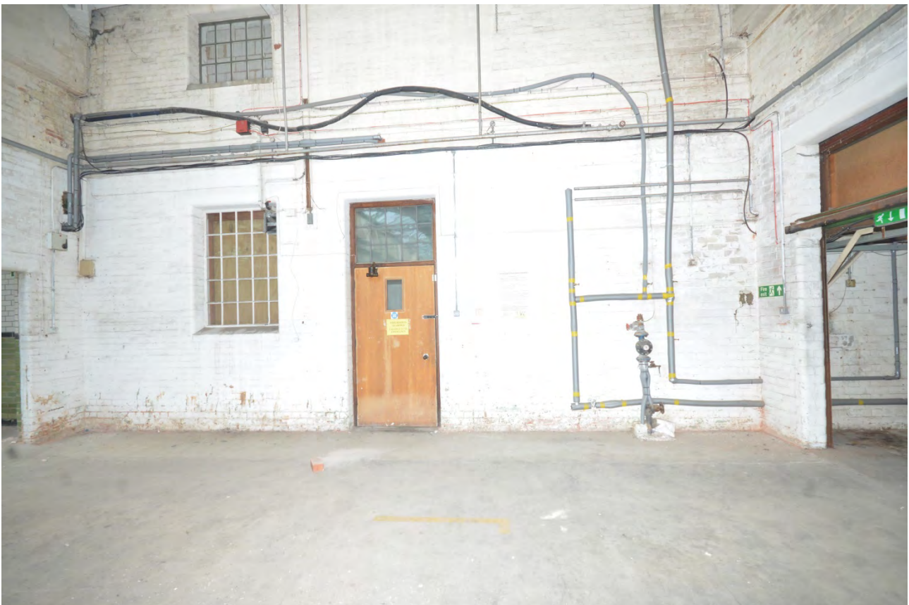
Plate 30: Door and windows to administration building in southeast wall of manufactory room 3
