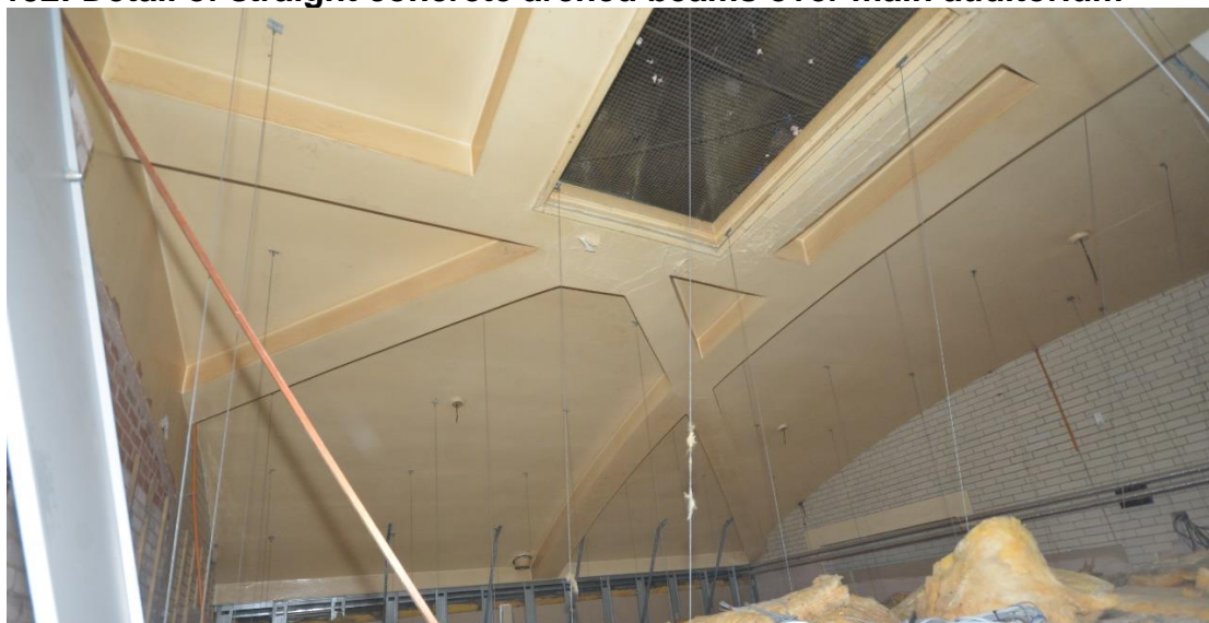
Plate 153: Detail of bracing formed by arched concrete beams, southwest of main auditorium
