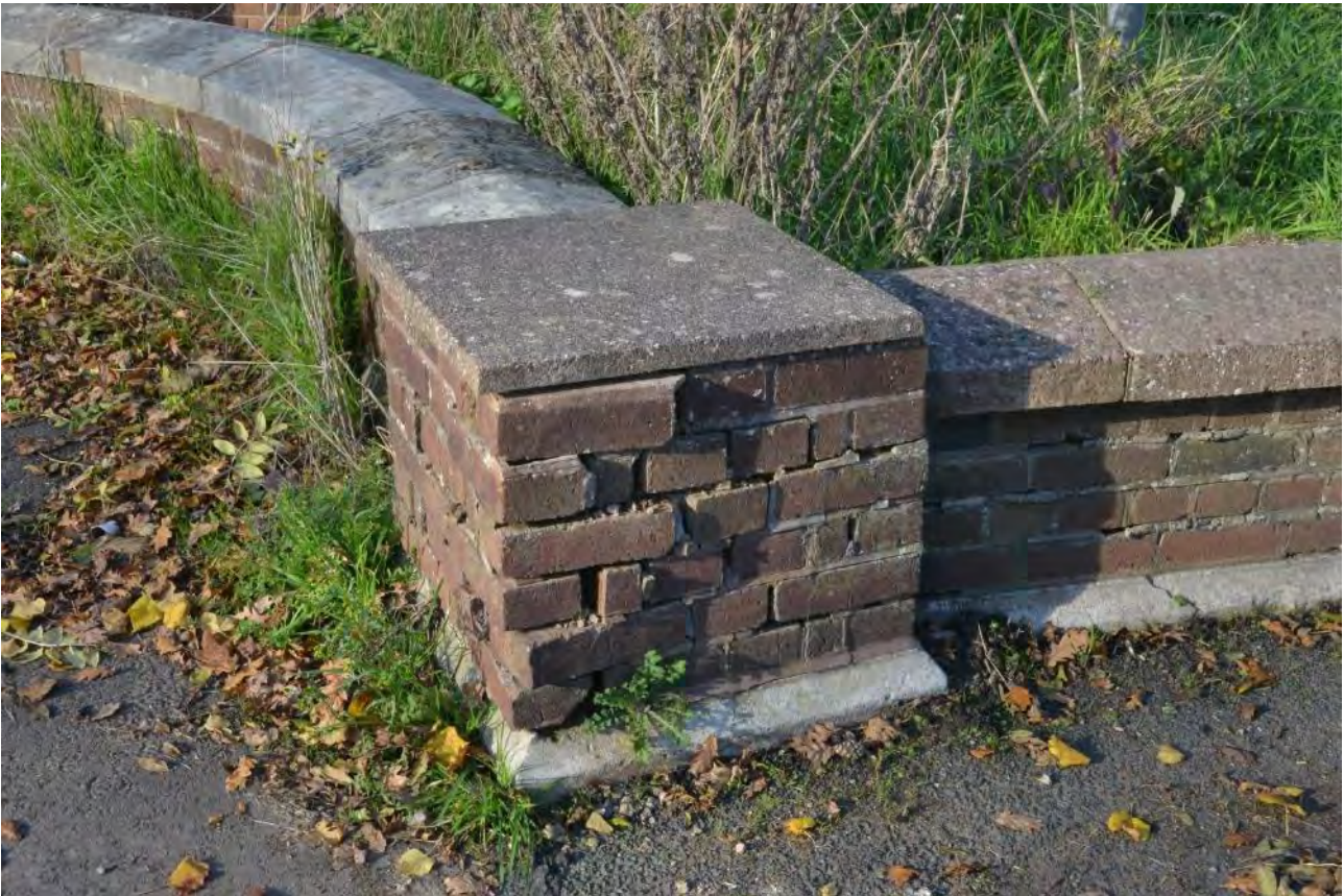
Plate 13: Corner of low wall to northeast of gate, showing collision damage
