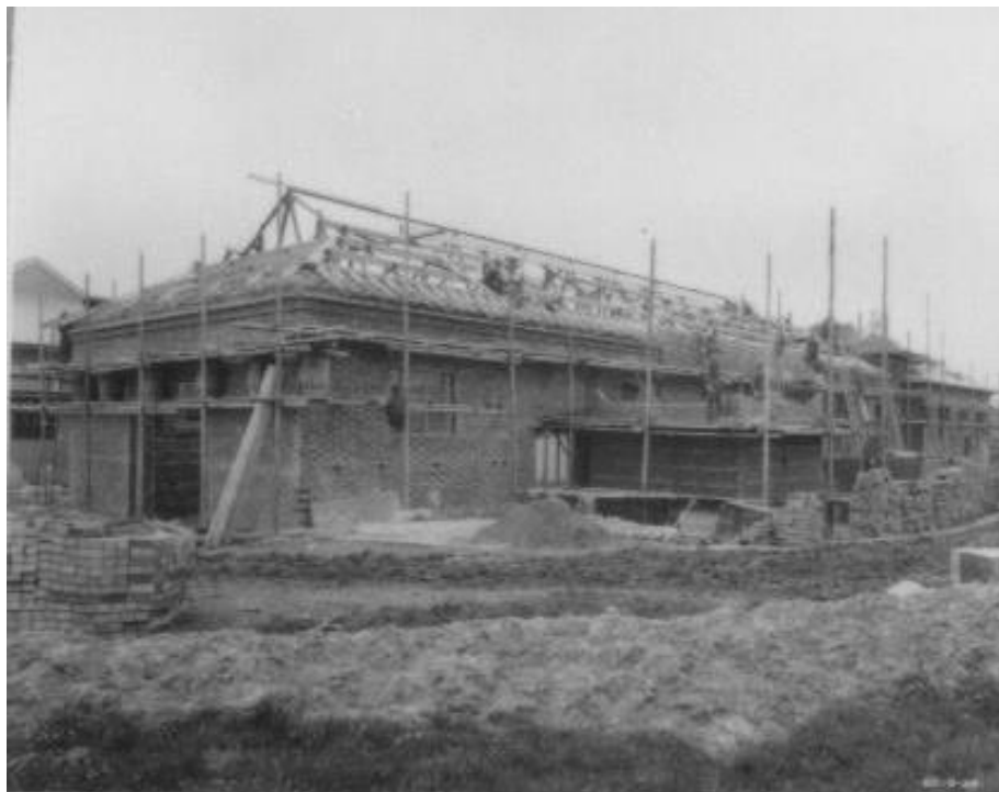
Figure 3: Boiler house and power house under construction, 1920s (Blue Bird Album, Romsley & Hunnington History Society)
