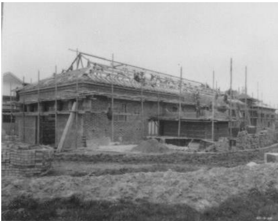
Figure 8: North aspect of boiler house and power house under construction, 1920s (Blue Bird Album, Romsley & Hunnington History Society)
